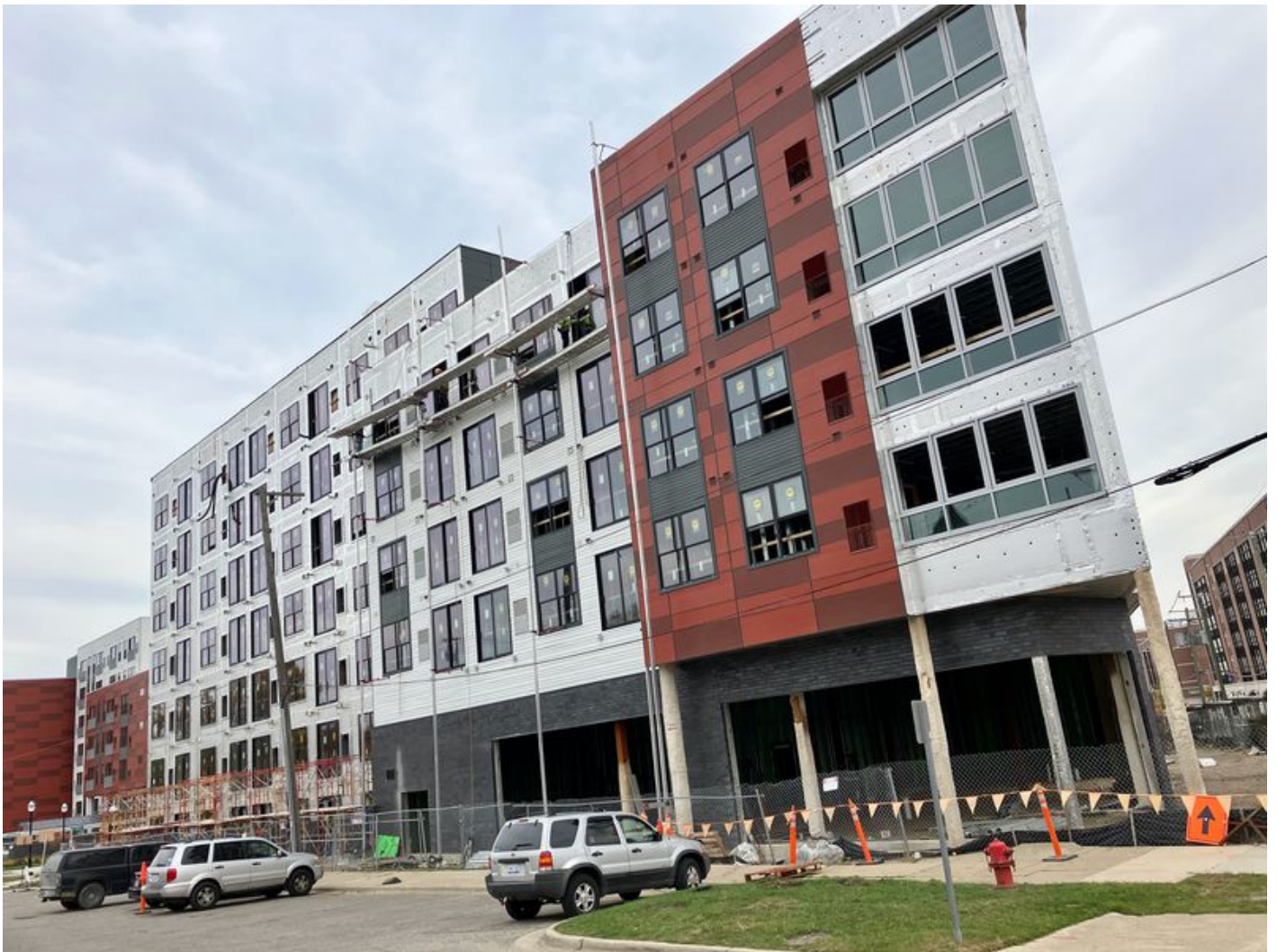
A second apartment building is under construction at the Beekman on Broadway development site in Ann Arbor on Oct. 24, 2022. Ryan Stanton | The Ann Arbor News
