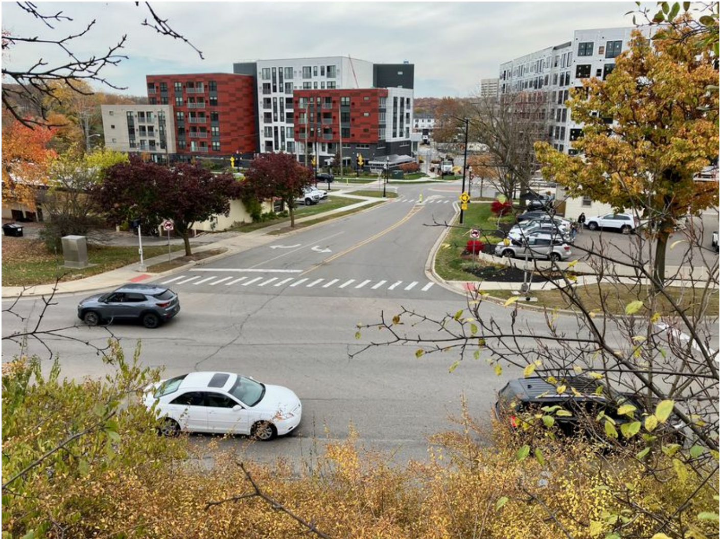
A second apartment building is under construction at the Beekman on Broadway development site in Ann Arbor on Oct. 24, 2022. Ryan Stanton | The Ann Arbor News
